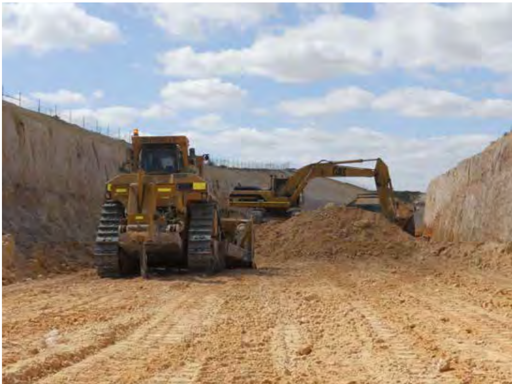
RJ Vincent won the Category 3 WA Earth Award for the Butler Rail Extension - Civil Works Project, one of five projects recognised for construction and environmental excellence in the 2012 Awards.
